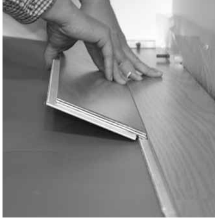
10. Position second row board at an angle and push down into place.
